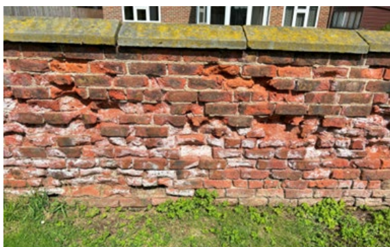
Brick wall with erosion
